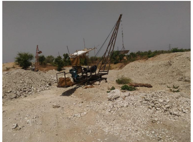
(Crane wire need to checked)
