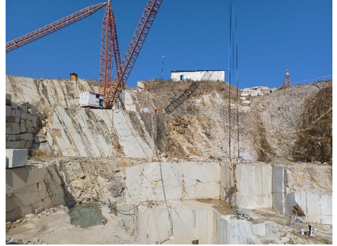
(Crane wire need to changed timely)
